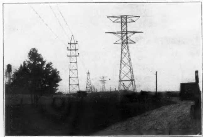
FIG. 20—TOWER LINE NEAR LINE OF N., L. & O. TRANSMISSION
